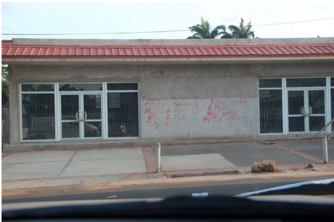
Image 3: Closing the building as a reaction to noncompliance with planning regulations (Arku 2016)
